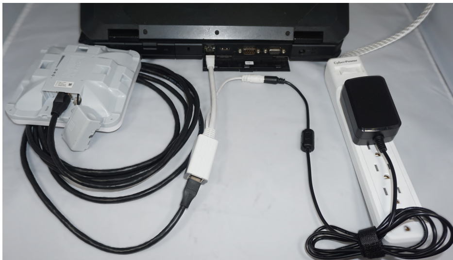
Figure 23: Shoreside Hardware Setup
