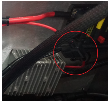
Figure 59: Navigation Fuse Location
